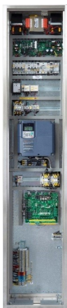
Quadro al piano (MRL)
